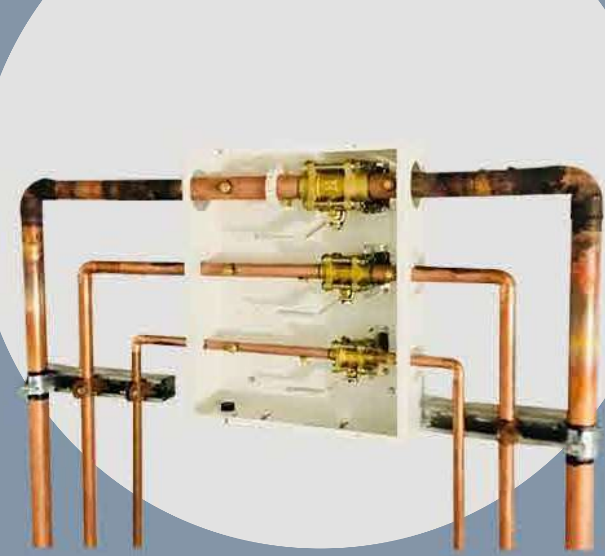
Central Oxygen Pipeline
